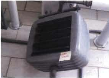
Modine Steam Unit Heater No Data - Painted over Location: Lavatory
