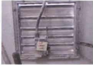
Lime Silo - Upper Motorized Louver/Shutter Model No. 2C831B 120 V; 0.21 Amp
