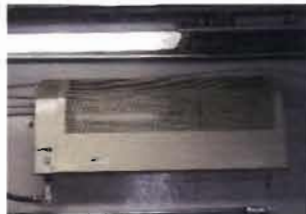
Chromalox Electric Unit Heater Cat No. HCH-501M 277 V; 1 Phase; 5000 Watts EF-8 - Lower Level Pump Area
