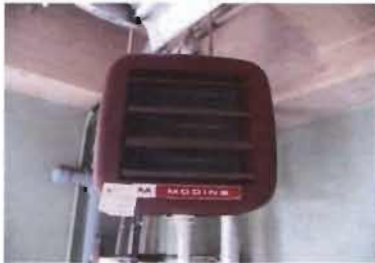
Steam Unit Heater Modine Model No. HS33S01 Serial No. SP011996 Location: Old Generator Room
