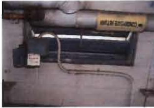
PFP - Fluoride Room Motorized Louver No Data
