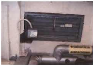
PFP - Hypo Room Motorized Louver No Data
