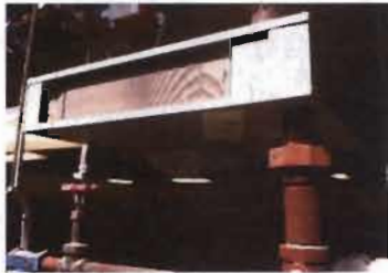
Trane Unit Heater Steam Location: Near Rear Entrance
