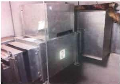
Exhaust Fan EF-2 Location: Pump Room Greenheck Model No. BSQ-80-3 Serial No. 06H26880 Belt: 4L-370R Includes intake louvers
