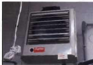
Lime Silo - Upper Dayton Unit Heater Model No. 2YU70 480 V; 10 KW; 3 Phase; 0.22 Amp
