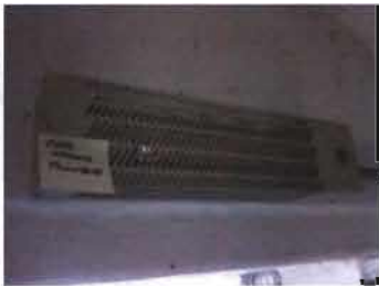
Electric Radiator Heater 24" Long; 120 Volt Model No. 3502-2861-000 207033541 Location: Fountain Pit Near Park
