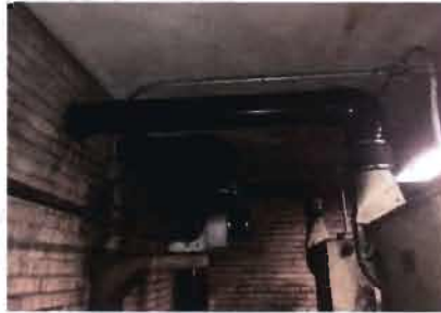
Carbon Room ductwork to be cleaned Annually
