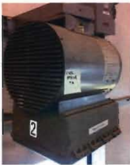
Electric Unit Heater - EUH-2 Marley Electric Heater Model No. W75041A MFG Code - L94 7.5 KW; 240 V; Single Phase Location: Pump Station
