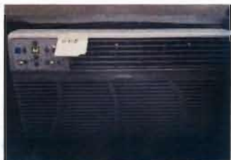
Feddgers Air Conditioner Window Unit Location: SCADA Room in Pump Station
