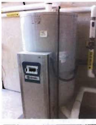
Automatic Electric Water Heater AO Smith Model DSE120A Serial No. 1301R000001 Item ID: 9500010810 120 Gals; 3 phase; 480 V; 7 Amp; 6000 Watt Location: In Membrane Area
