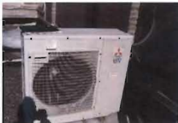
BMP - Rooftop Units Mitsubishi R410A, Mr. Slim Split Unit Matches to Foreman's Office Model MXZ-3A30NA 208/230 V; 1 Phase S/N: 61901162B
