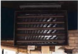
PFP - Garage Trane Steam Unit Heater Model No UHSA-060S-8C-AAE S/N: D91H08896
