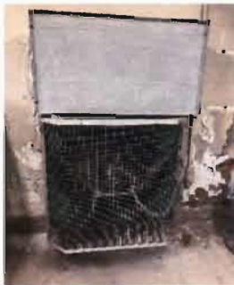
Exhaust Fan No data Available Location: Former Chlorine Room in Pump Station
