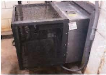
Cook Ventilator EF-4 Model No. 200XMW Serial No. 076SE49822-00/0000701 0.5 Hp; 3100 CFM; ODP Motor 465 V; 1725 RPM February, 2013 Sdesign SP: 0.38 Location: ACH Feed Room
