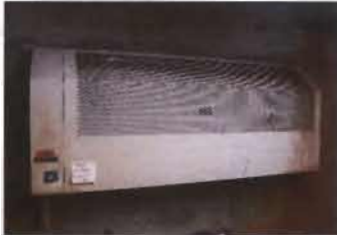
PFP - Sludge Building - Lower Floor Chromalox HCH-501 172PP Electric Unit Heater Wall Mount 480V; 5000 Watt; 3 Phase
