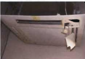
SCADA Room Split Unit
