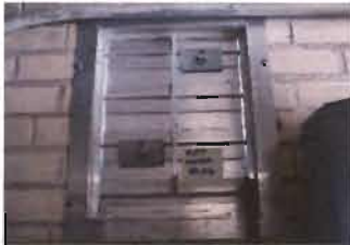
Metering Building Gravity Damper - One No Data
