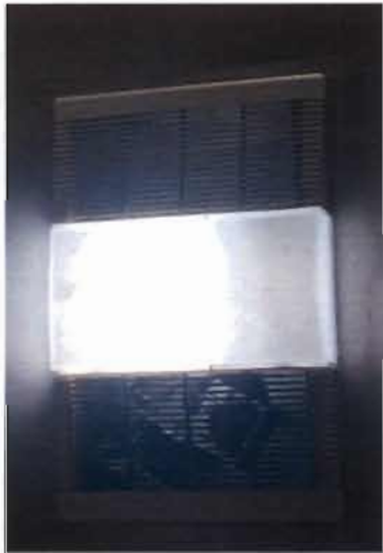
Carbon Locker Room One Vent Fan in Men's Room No Data
