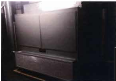
Trane Electric Heater Model: TWE180E300AA Serial No: 12204XCYWA Date: 5/20/12 Location: Electrical Room
