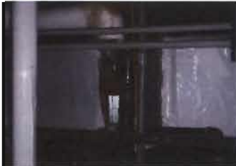
Filter Gallery Steam Heat Exchanger 23 Tube Replaced in 2018
