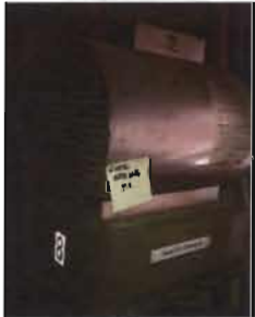
Electric Unit Heater - EUH-8 Marley Electric Heater Model No. W50041A Corrosion Resistent/Washdown MFG Code - L94 5 KW; 240 V; Single Phase Location: Pump Station
