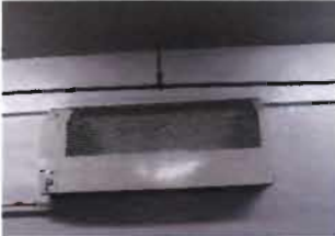
Chromalox Electric Unit Heater Cat No. HCH-501M 277 V; 1 Phase; 5000 Watts EF-7 - Lower Level Pump Area
