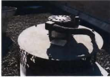
Direct Drive Vent AO Smith Model No. 323P672 115 V; 1.2 Amp (Restroom Vent)
