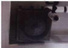
PFP - Basement Trane Unit Heater Model No. UHPA-102P-4A-BAD S/N: D911H08903 Near the Zinc Feed
