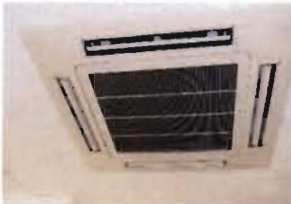
Main Lab Area Split Units
