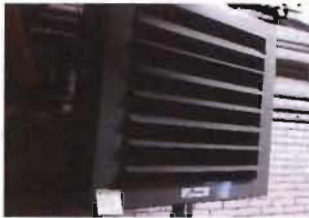
Steam Unit Heater Modine Hydronic Unit Heater Model No. HSB165S01 S/N: 30104407-3969 1/3 Hp; 115 V, 4.6 Amp Location: Basement Near Old Pump 3A/3B
