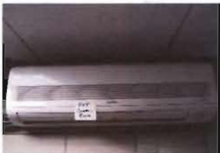
Control Room Sanyo Model KMHS0972 S/N: 0084193 8522134476000 230 V; 0.15 A; One Phase Tied to CWH3172 Sep-09
