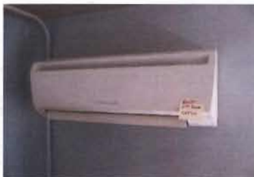
Mitsubishi Heat Pump, Split System Model No. MSZ-A12NA Serial No. 6004080-T 208 V; 1 Phase Location: Foreman's Office
