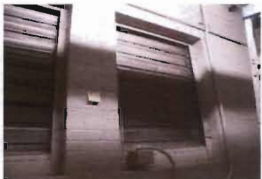
Two (2) Motorized Louvers 40" x 30" No Data Near No. 10 Sed Basin
