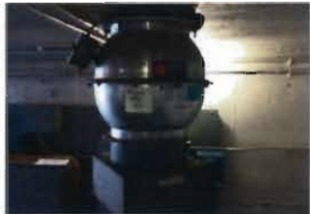
Loren Cook Ventilation Fan High Temperature exhaust Model: 10CV17D 20 A Breaker, 115 V; 1725 RPM; 1/6 HP S/N: 289S6479440000007010601
