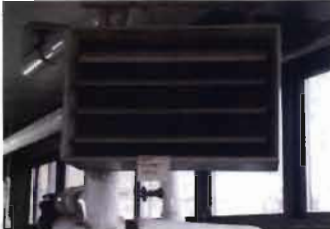
Filter Deck Trane Steam Unit Heater Model No. UHSA-042-8C-AAC S/N: Painted - No Data
