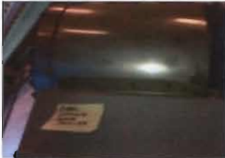
Electric Unit Heater - EUH-5 Location: Cool Spring Gate House TPI Corporation Model No. P3P5505 43WD501 480 V; 5 KW; 3 phase
