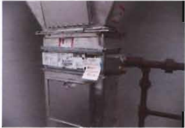
Trane Coil Type Heat Exchanger Coil Type: NS Sigma Flo Serial No. H12E04663 Order No. D2T823A Location: Carbon Room
