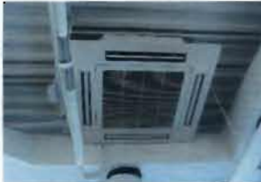
Water Quality Supervisor Office Split System
