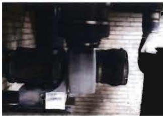
Carbon Feed Room Blower No Data
