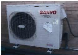
Split Unit on Roof Sanyo R410A Model C2472 S/N: 0044012 85221344675000 230 V; 10.8 Amp; single phase Date: 4/11
