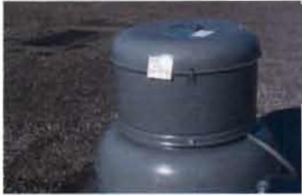
Cook Ventilation Unit EF-7 Model No. 120ACE 120C3B S/N: 076SE 49822-01/000-4401 0.25 Hp; 650 CFM; 115 V; 1 Phase Jan-13
