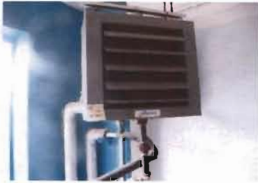
Hydronic Unit Heater Modine Model No HSB86501 Serial No. 38014008-1638 1/8 Hp; 115 V; 1 Phase; 2.3 Amp Shop Area - 2nd Floor
