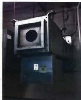
Exhaust Fan - EF-2 Location: Pump Room Greenheck Model No. BSQ-70-4 Serial No: 06H26878 Belt: 3L-360
