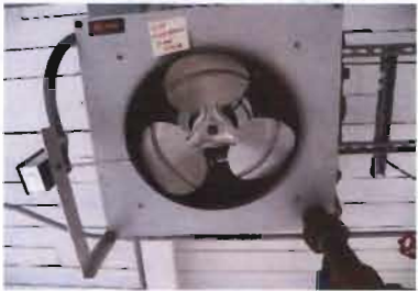
Steam Unit Heater Trane Model UHPB0801TAA4000004B Serial No. F12E32494 1200 CFM; 80,600 BTU/Hr Output 115 V; 1 Phase; 2.1 Amp Location: Membrane Feed Pump Room
