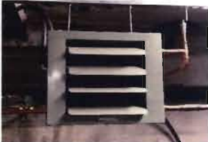
One Hydronic Unit Heat in basement of Gate House Modine Model No. 47SB01SA Serial No. 39105018-5464 1/12 Hp; 115 volt; 1.7 Amp
