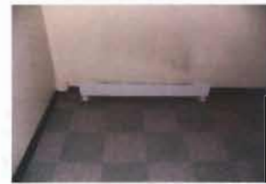
Basement Staircase Floor Radiator
