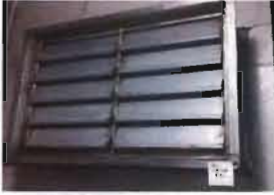
Gravity Louver Location: Pump Room
