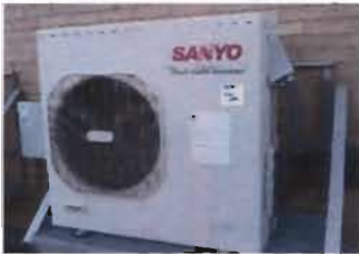
Split Unit on Roof Sanyo Flexi Multi Inverter Model CMH 3172 S/N: 0012193 85221344585002 230 V; single phase Date: July 2009
