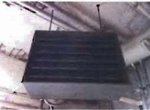
Steam Unit Heater Trane Model UHSA 10058AAAE Type 136-108-01 S/N: D82K4571 Location: BPS Basement near Old Pump 3A/3B
