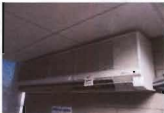
Control Room Sanyo KHS3672R S/N: 0057393 230 V; 0.5 A; 1 Phase Tied to C3672R
