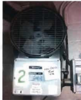
Electric Unit Heater - EUH-2 Location: Pump Room Chromoloz Model No. HD3D-750 Serial No. 004-305492-023 480 V; 7.5 KW; 3 Phase
