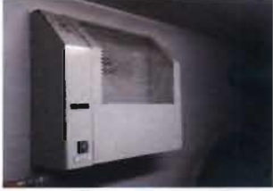
Chromalox Electric Unit Heater Cat No. HCH-051M 277 V; 1 Phase; 500 Watts EF-6 Valve Nook - Lower Level
