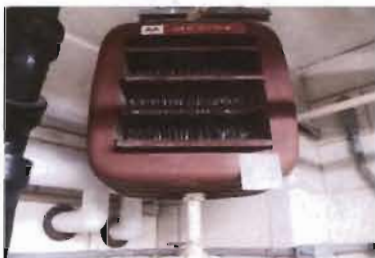
Steam Unit Heater Modine Model No. HS33501 Serial No. SP0011996 Location: ACH Feed Room
