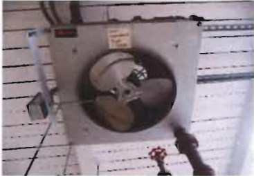
Steam Unit Heater Trane Model UHPB0801TAA4000004B Serial No. F12E32493 1200 CFM; 80,600 BTU/Hr Output 115 V; 1 Phase; 2.1 Amp Location: Membrane Feed Pump Room
