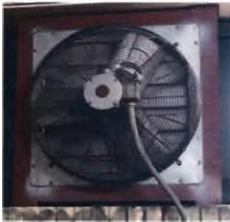
Dry Chemical Storage area Exhaust Fan
