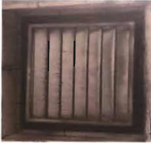
Interior louvers to be cleaned annually
