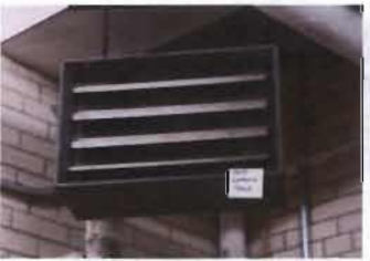
Loading Dock, Near Elevator Trane Steam Unit Heater Model No UHSA-038S-8C-AAC S/N: D91H08890
