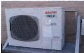
Split Unit on Roof SanyoR410A Model C3672R S/N: 0007092
