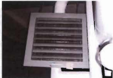
Hydronic Unit Heater Modine Model No. HSB193SB01SA (Year: 2018) Serial No. 43104517-1284 1/3 Hp; 115 V; 4.2 Amp Near Sed Basin No 7 South Side
