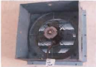
PFP - Hypo Room 18-inch Exhaust Fan No Data
