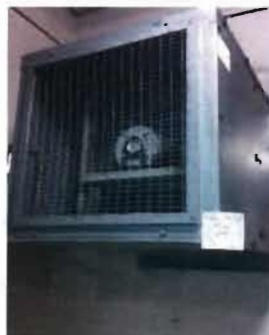
Exhaust Fan - EF-1 Location: Pump Room Greenheck Model No. SE2-16-417-A3 Serial No: 06100123 Direct Drive
