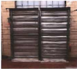
Actuated Louvers Quantity: 4
